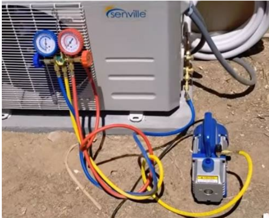
Figure 2: Example of a vacuum pump connected to a mini split unit with a gauge set.
